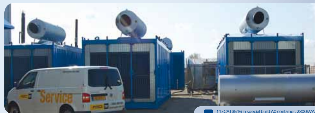
11xCAT3516 in special build A0 container, 2300kVA
